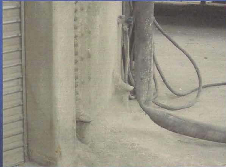
Bolted steel silo leaking material
